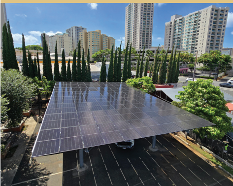
COVERED PARKING FOR SHADE & POWER
