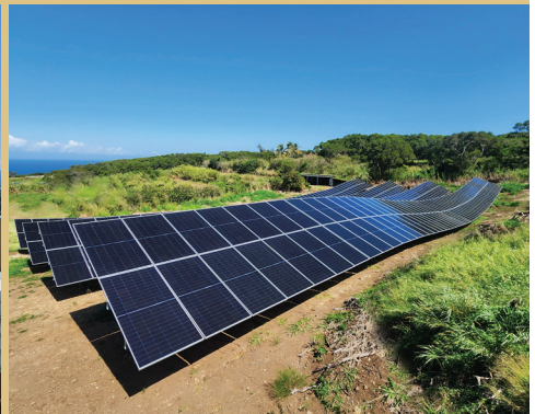
SOLAR ARRAY TO UTILIZE IDLE GROUNDS
