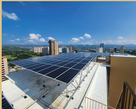
ELEVATED SOLAR ARRAY ON FLAT ROOFS
